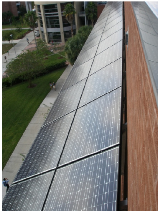
Figure 7 – Solar Panel Outside UCF Engineering Building
