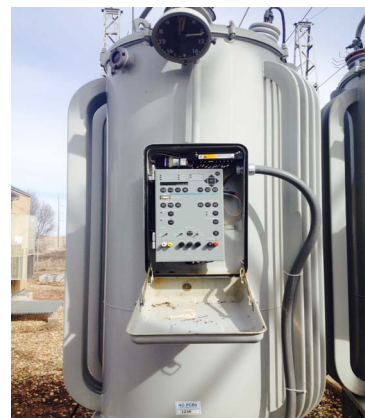
Figure 1. Sioux Valley Energy Voltage Regulator
